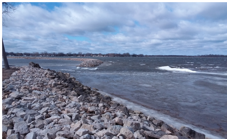
Breakwall One Week After Construction
